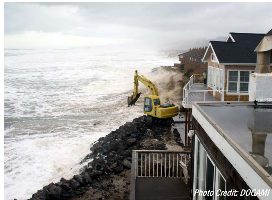
Damage from storm waves during a “moderate” event at Neskowin, Tillamook County.
