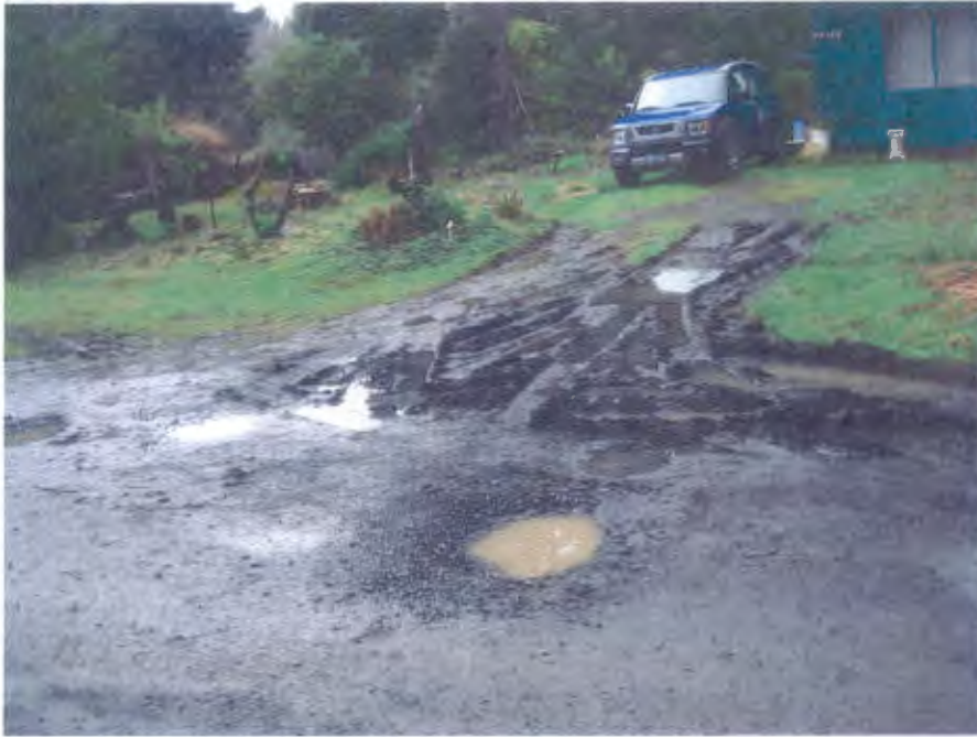
Poor road drainage inundates driveway
